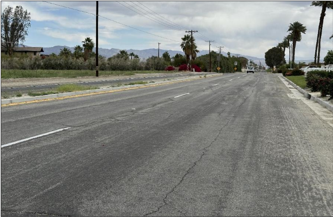
Figure 5-5 Avenue 50 segment with cracking in asphalt from Verano Drive, facing northeast.
